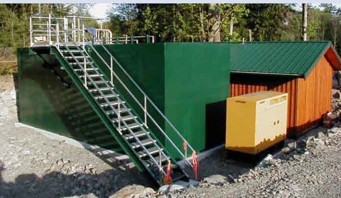
25,000GPD (100m 3 /d) packaged USBF™ WWTP. Located directly on a golf course, attesting to the minimal noise and non-odorous nature of the process.
