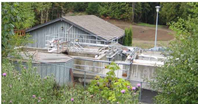
32,000GPD (120m 3 /d) Class A+ USBF™ WWTP. Water reused for nearby aquifer recharge.
