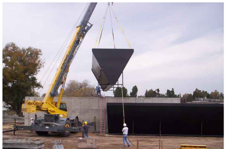
Installation of the USBF™ filter into IMGD (4,000m 3 /d) municipal USBF™ WWTP.
